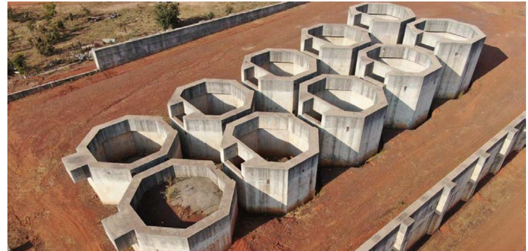
Rougher Flotation Cell Pedestals
