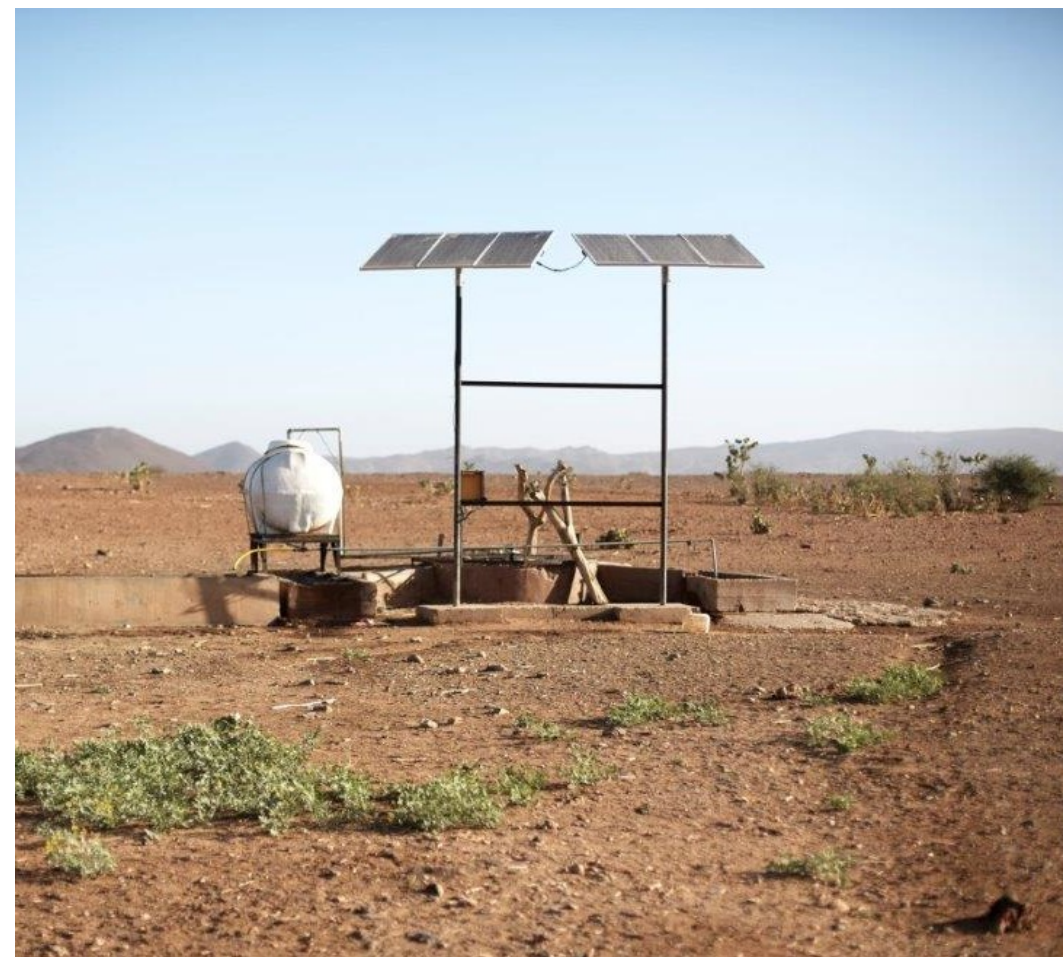
Solar water pump in Mauritania
